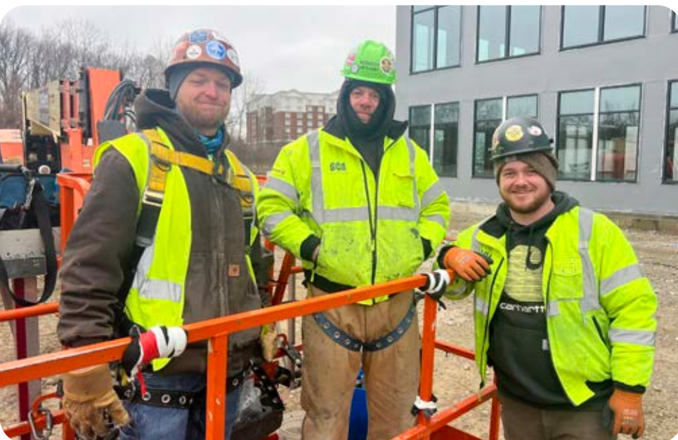
Local 181 members Roy Hall, Matt Brockett and Dakota Page working for Carroll Glass at Project Visibility.
