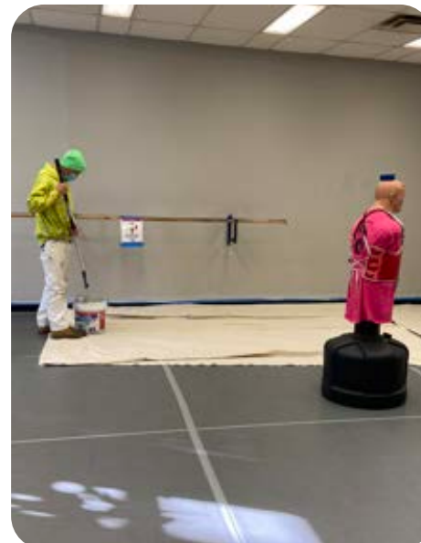
Daniel Brown and Timothy Lansdale, fourth-year apprentices, paint the St. Bernard Community Center in Cincinnati.
