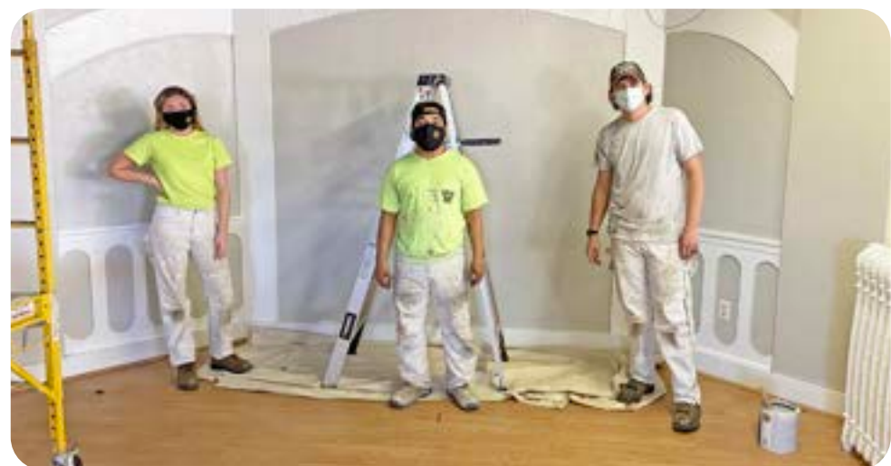
PHOTOS: COURTESY OF IUPAT DC 6 Dayton Union Hall getting an all-around overhaul with a new roof and apprentices taking the time to repaint the interior of the building. Thank you apprentices!
