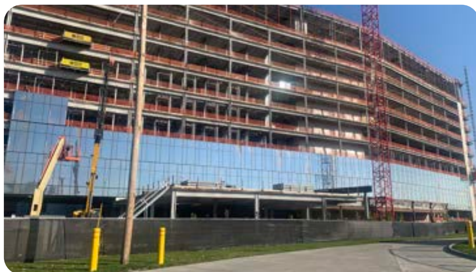
Harmon Glass crew steady at work on the Cleveland Metro Hospital Downtown.
