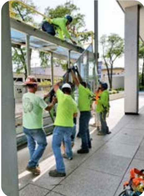
Interstate Commercial Glass and Door crew working on the Hylant building in downtown Toledo.
