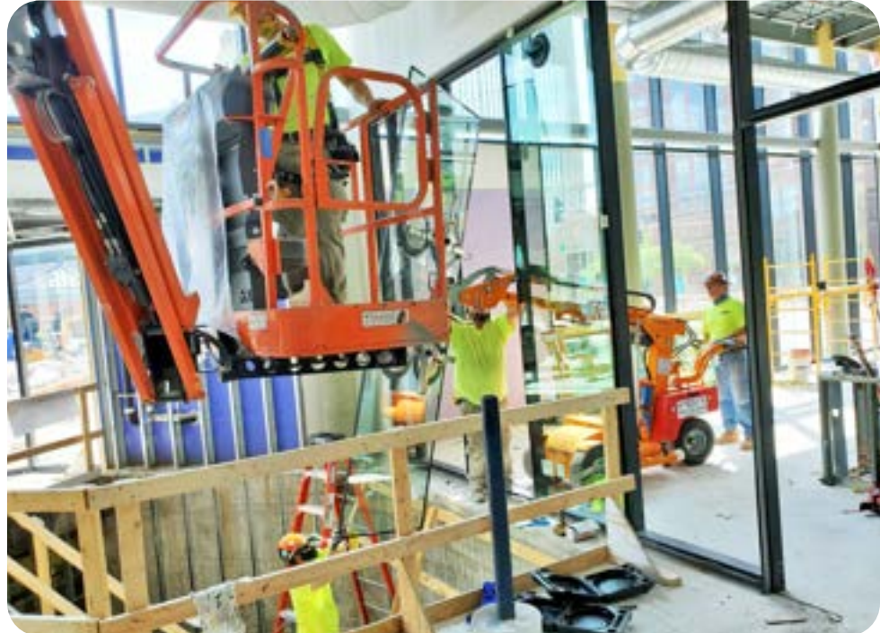
Toledo Mirror and Glass crew setting a unit at Imagination Station in downtown Toledo.
