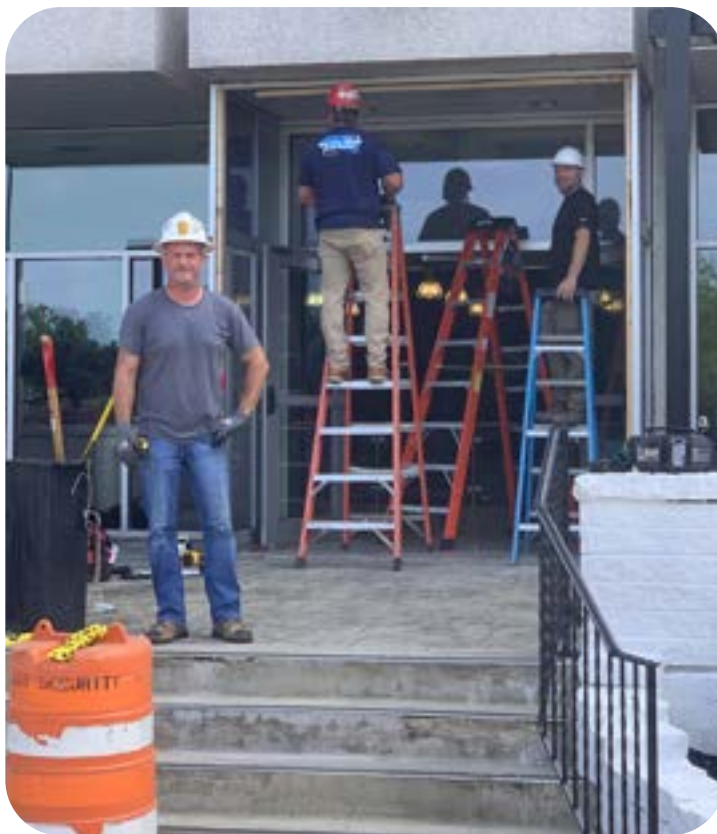
From left: Local 847 members Brian Griffiths, Ben Canfield and Hank Haddle, working for Warren Glass Glaziers on the entrance to the Lordstown Motors Plant.
