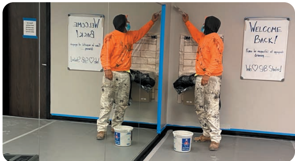
Fourth-year apprentice Timothy Lansdale helps spruce up St. Bernard's Community Center in Cincinnati by giving it a new coat of paint.
