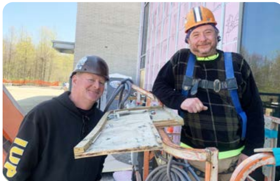
Local 181 Glaziers, Mike Michalk (Left) and Nick Beach (Right) working for RC Glass at University Hospital Avon office.
