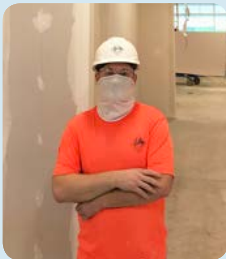
Finisher Scott Brumfield with Valley Interiors working at Chase Bank headquarters in Lewis Center.
