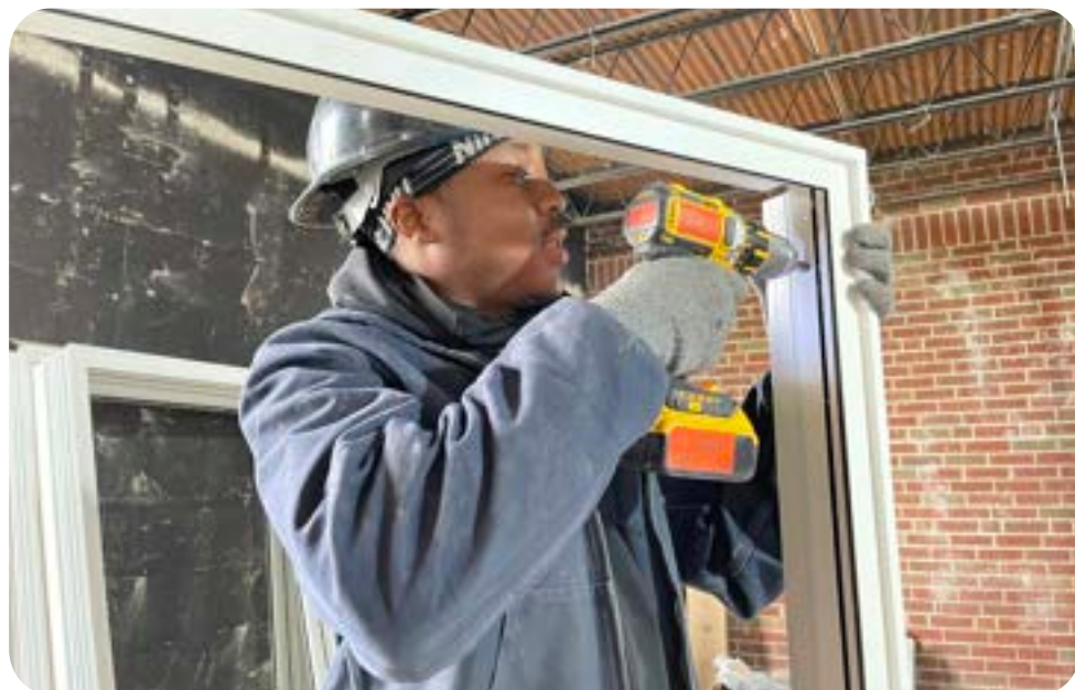
Local 181 Glazing Apprentice Brian Walker working on Center for Pastoral Leadership framing/sash.
