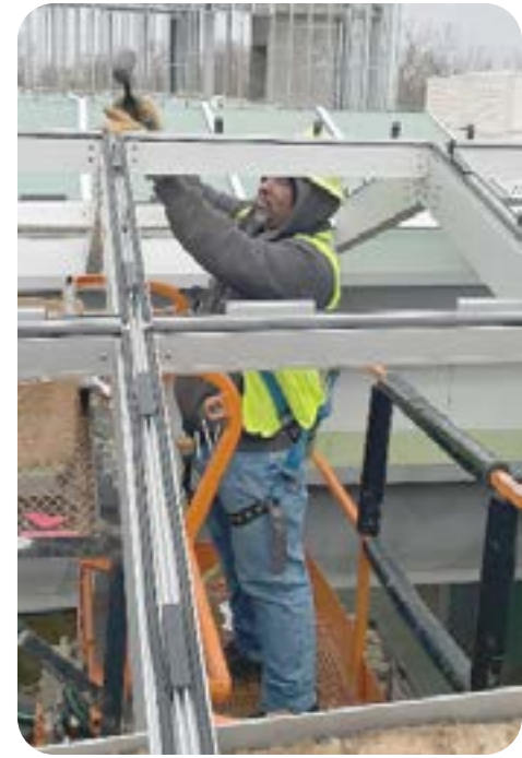
Glaziers Local 1162 journeyman W.J. Smothers, working for RC Glass, installs a skylight at the LG plant in Ravenna.
